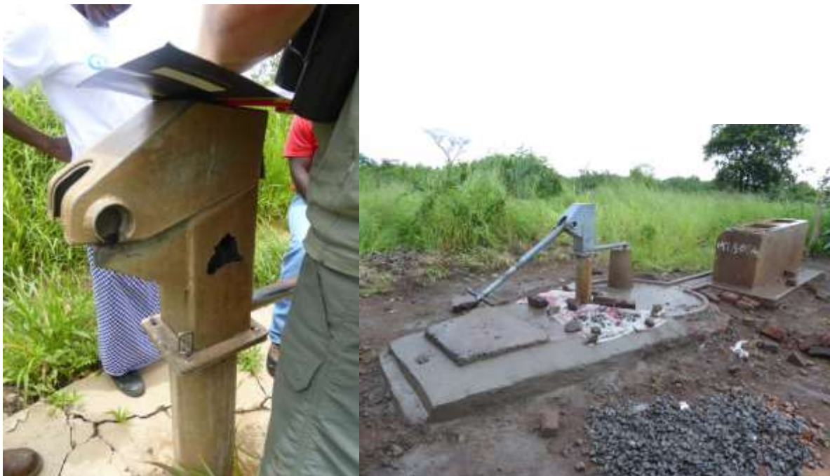
Figure 10 Damaged head and civil improvements at 15. Chibangalala
