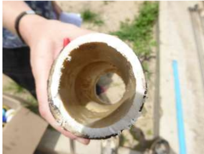
Figure 3. Misaligned pipes at 2. Jangavya.
